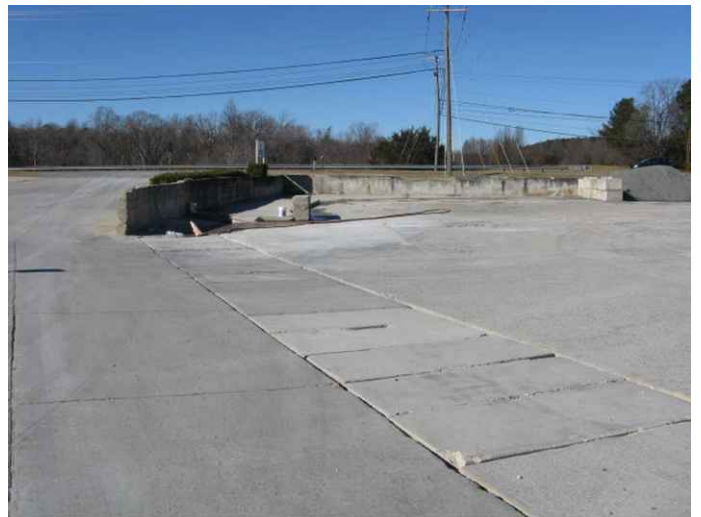
Underground Sediment Collection System
